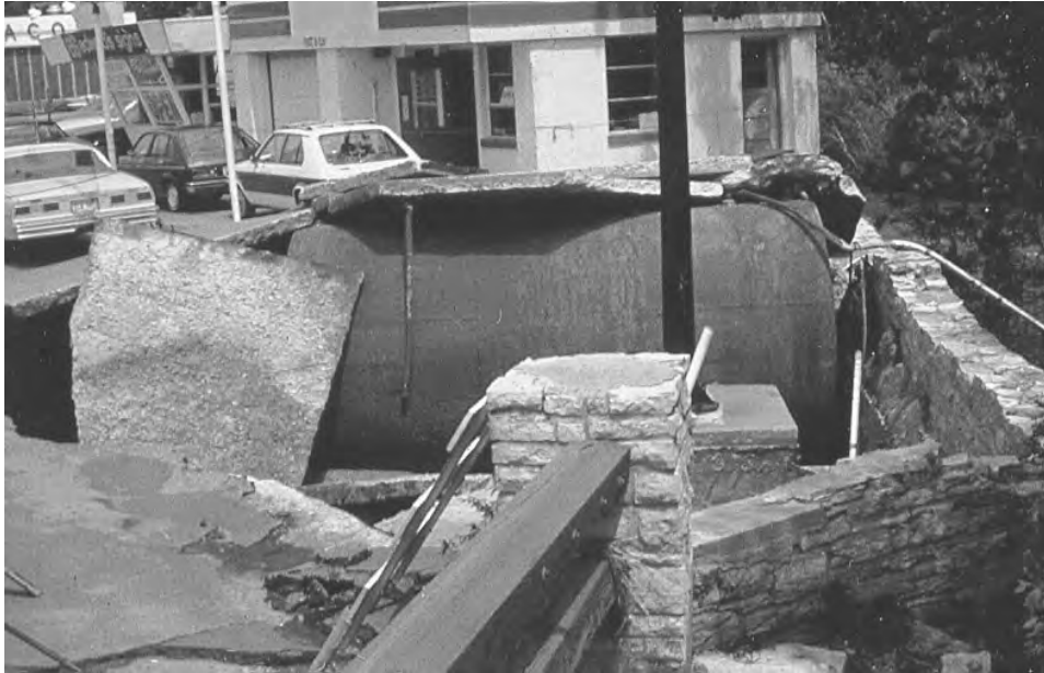
Figure 3.2.3.1A: Tank lifted by buoyancy forces
